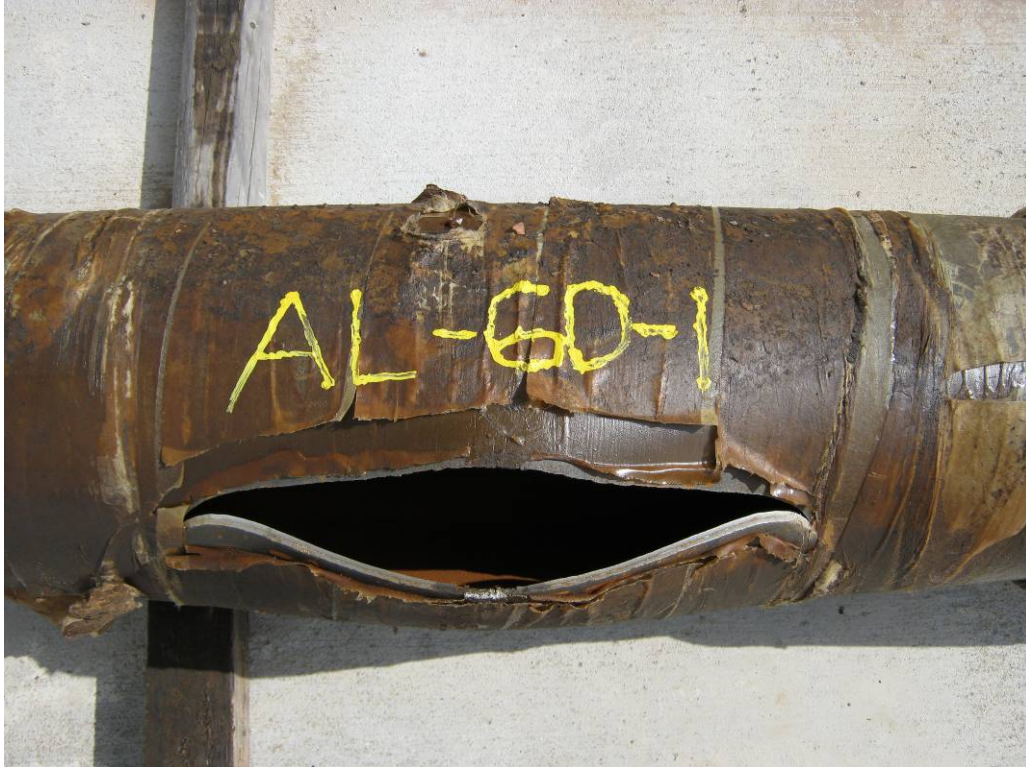
Figure 5 – Photograph of Failure Location, 60% Corrosion Sample
