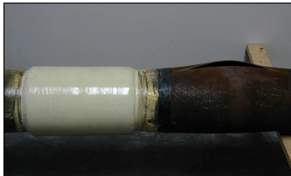
Figure 4.2 12.75" OD pipe with ruptured section adjacent to wrap.
