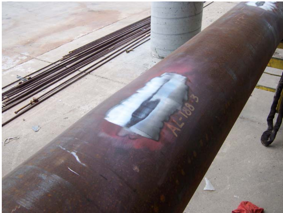
Figure 4 - Gouge removed by grinding
