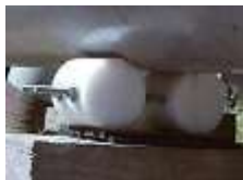
Pipe support and insulation system
